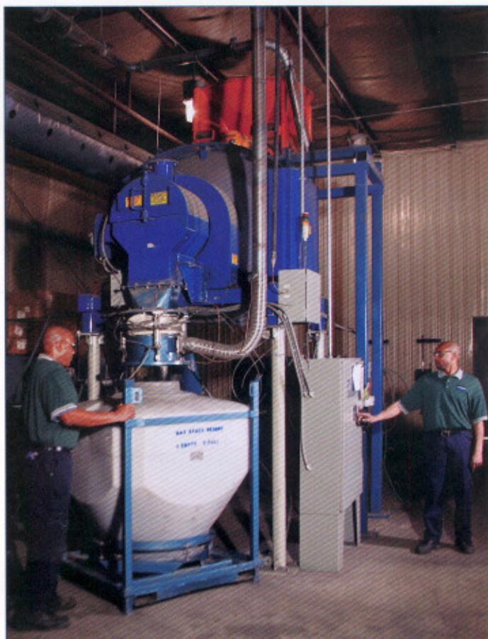
Munson rotary batch mixer processes 2500 kg batches of powdered metal components. Raw powder ingredients enter from surge hopper above and blended powders discharge into intermediate bulk container below.
